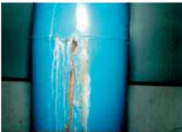
Picture 3. A corroded AISI 304L main pipe from a water extraction company that leaked after 1 year because backing gas was not used.
