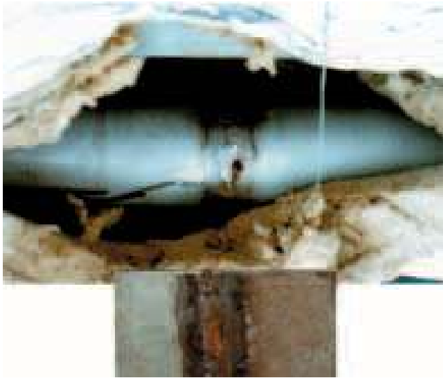
Picture 2. Leaking AISI 316L cooling water pipe because backing gas was not used. The burnt root penetration side can be seen on the lowermost illustration.
