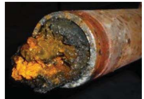
Figure 3: Steel pipe totally clogged by corrosion products (photo: MIC Europe private company)
