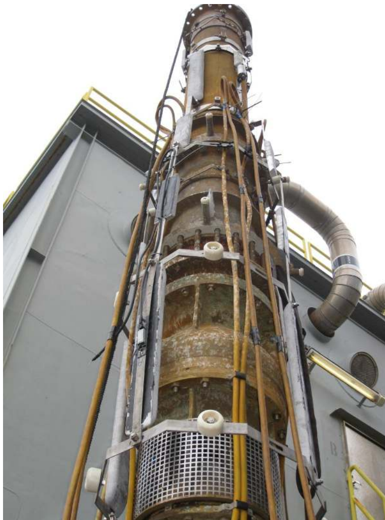
Figure 5: Picture of hanging anode construction. Above: anodes and potential control unit are fixed on riser with bracelet construction. Three rows of anodes are hanging on this bracelet. Small anode left: Zinc-reference anode. Below: pump inlet. Ten sided stainless steel rings with Nylon centralizers keep the construction tight in the caisson.
