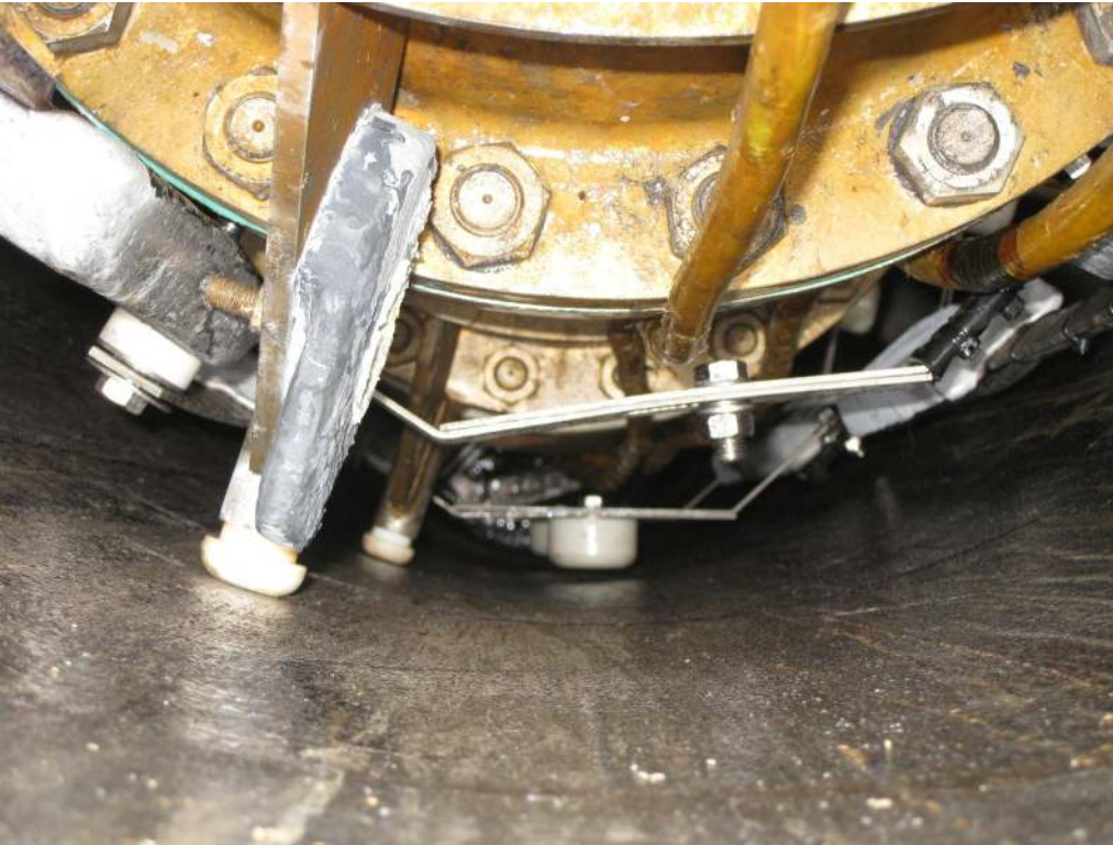
Figure 6: Anodes hanging in the annulus. Note the robust but flexible construction with 10-sided stainless steel rings and Nylon centralizers.
