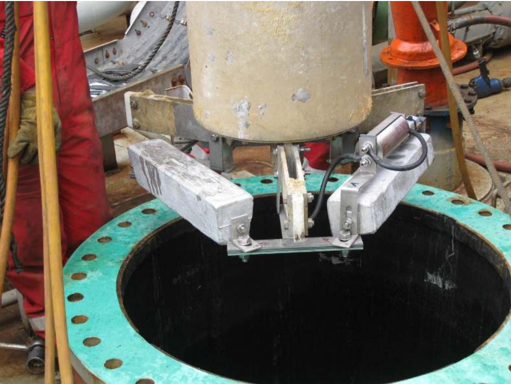
Figure 7: Tank anodes below the pump motor. The stainless steel cylinder is the subsea enclosure with potential control unit. Behind the enclosure a Zinc-reference probe can be noted.
