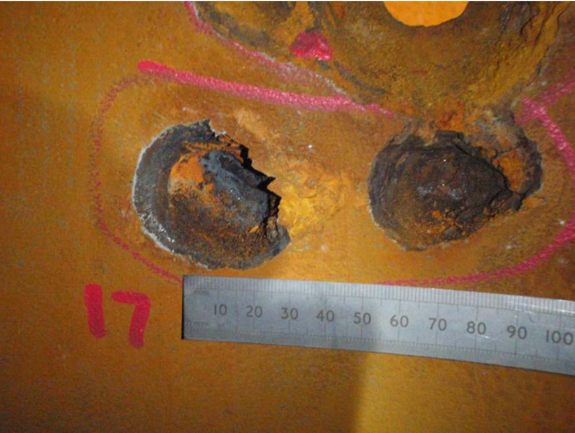
Figure 1: Holes in the caisson within two years lifetime.
