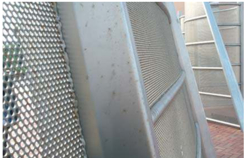
Picture 4. Rust pits showing on the design's posts.
