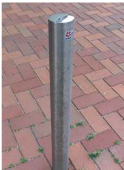
Picture 1. A stainless steel AISI 316 post, where all but the polished cap is corroded.
