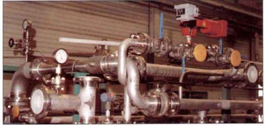
Pipelines in 316L
