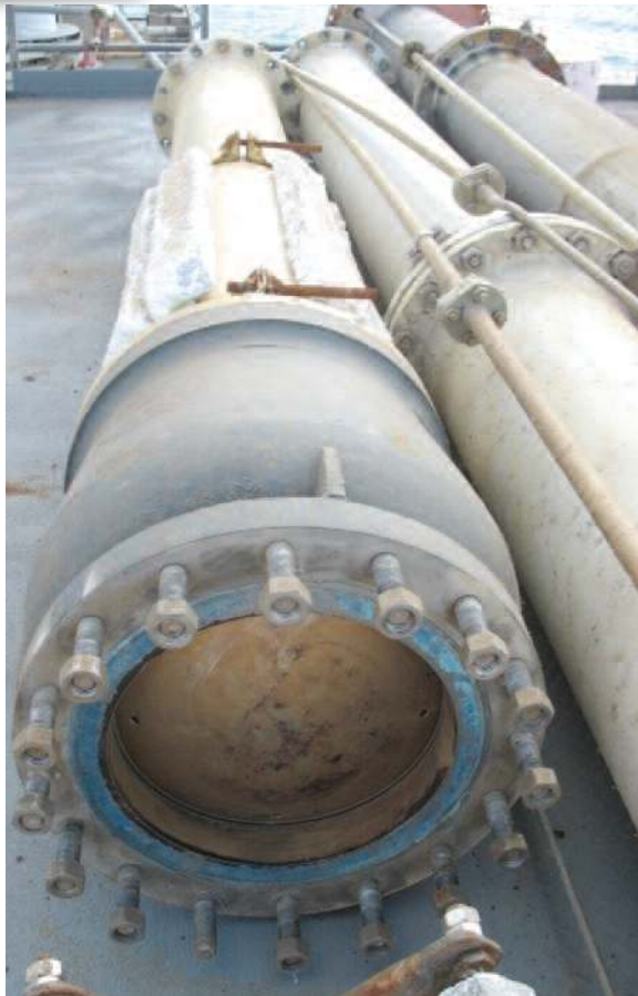
Fig. 6. Cast duplex stainless steel pump flange connected to duplex SS riser. Sacrificial anodes connected to the duplex stainless steel riser.
