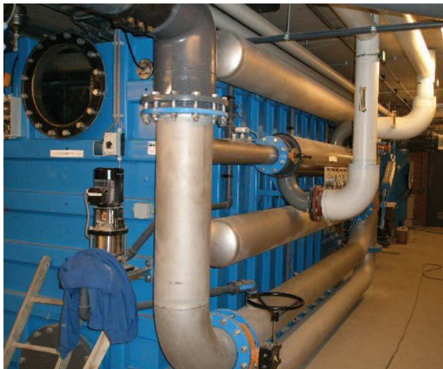
Fig. 3. Stainless steel sand bed filters used for cleaning swimming pool water are also protected using intelligent cathodic protection (photo by Innomet B.V.).
