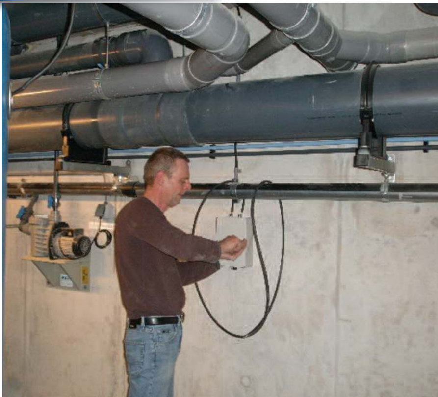
Fig. 1. Installation of an intelligent cathodic protection system in a stainless sand bed filter (photo by Innomet B.V.).
